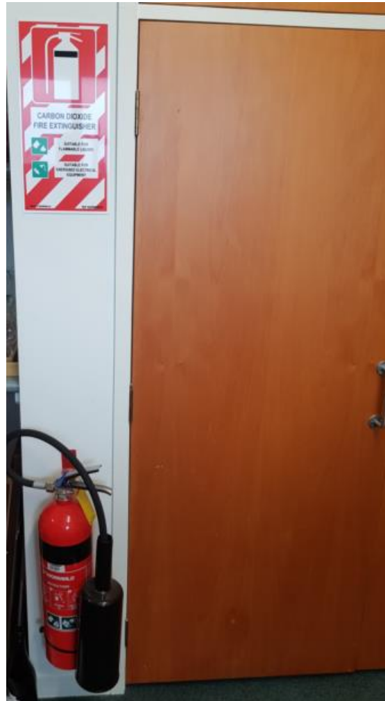
First Extinguisher inside the Sacristy
